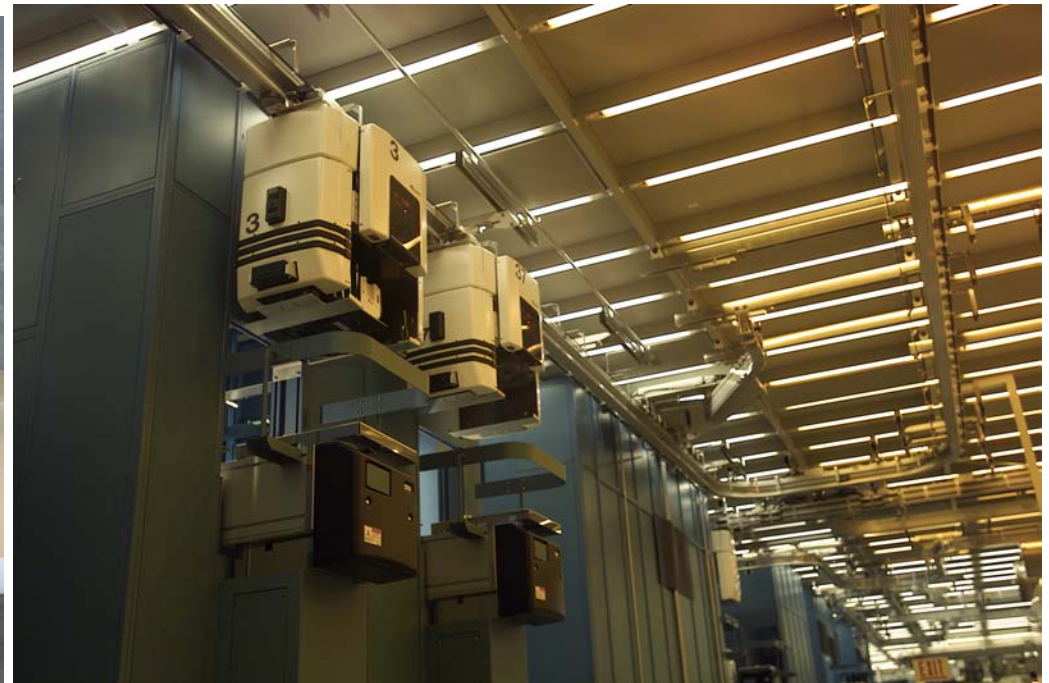
Overhead rail transport of wafer cassette
