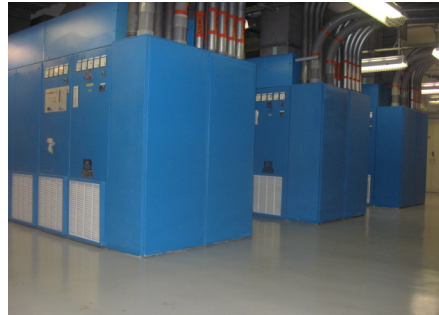
Uninterruptible Power Supply (UPS)
